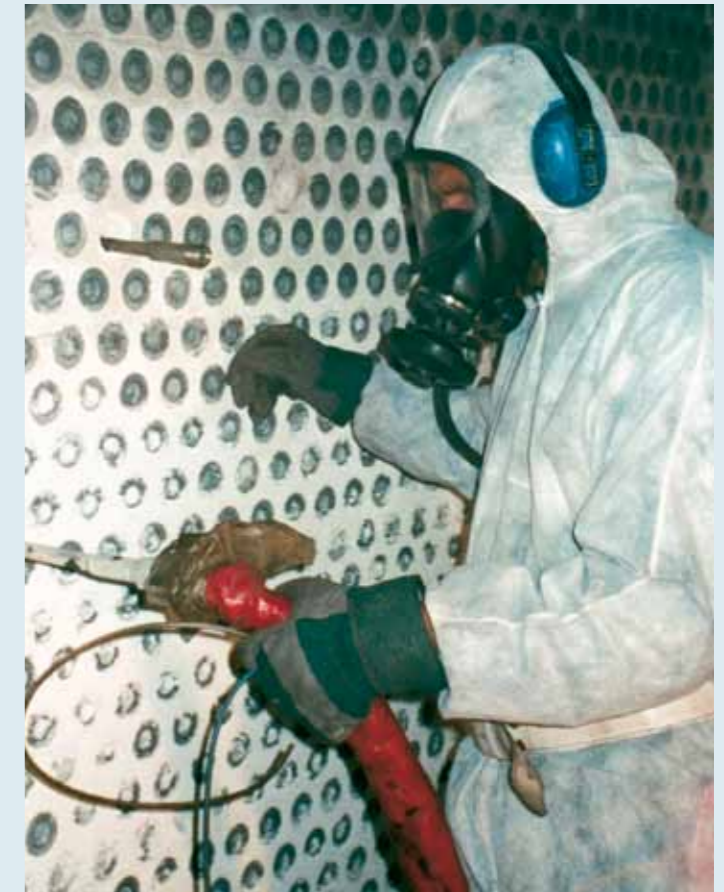
In some cases, gas masks are highly recommended – e.g. when cleaning heat exchangers and harmful materials are blasted loose.
